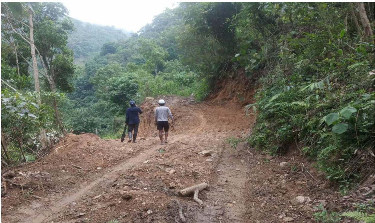
Figure 6.17: Excess road from powerhouse to surge tank.
