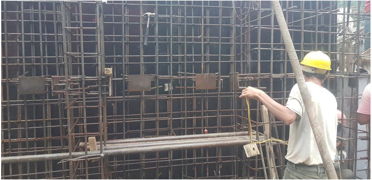
Figure 6.7: Installation of first stage embedded parts at undersluice gate and stoplog groove.
